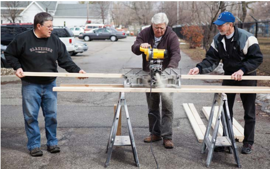
▲ Tom Weintraut, from left, Steve Rasmussen and Bill McGuire work together to build a shelf during the Saint Meinrad Day of Service in Indianapolis.
